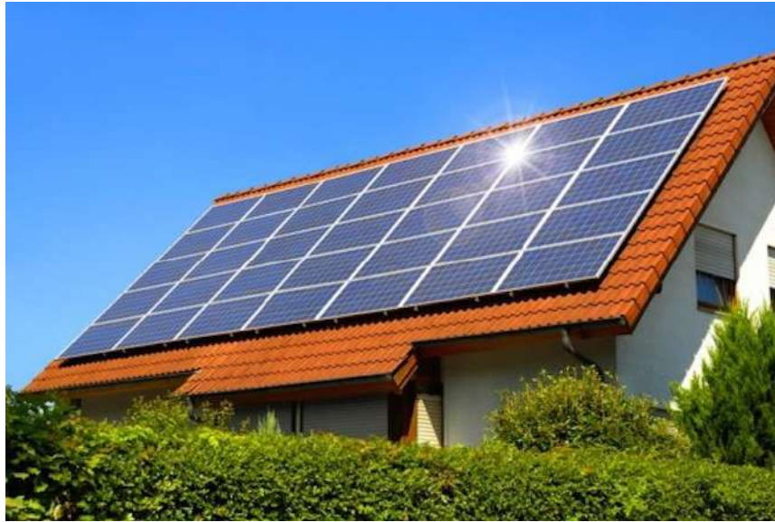
Figure 7.10: A rooftop array of photovoltaic cells.
