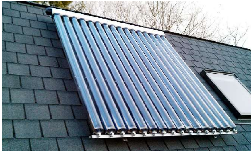
Figure 7.13: A rooftop solar thermal array for domestic water heating.
